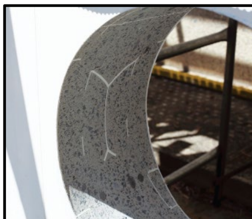
Fig 12. SCC concrete free of voids ( image extracted from Dincel literature )
