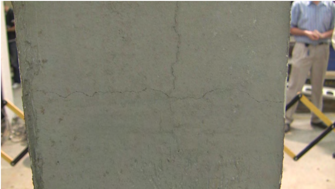
Figure 5.14 (e) Close Up View of Crack at X = 1150mm
