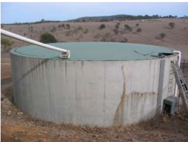
Photo showing cracked and leaking concrete water tank
