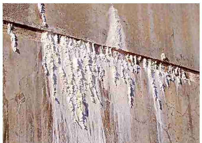
Photo showing carbonation at leaking concrete wall joint
