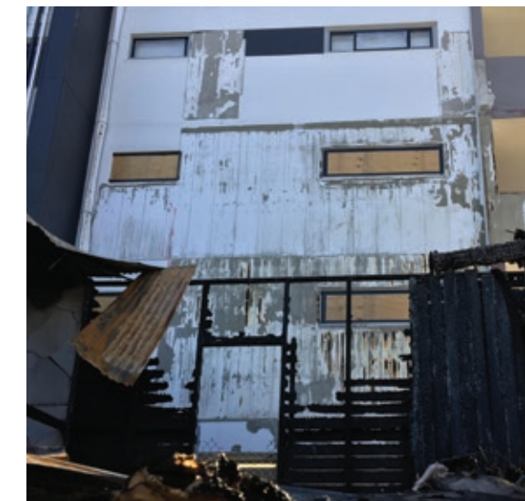
The Dincel panels polymer skin after the QLD fire event in Mar 17 remained intact, ready for re-rendering.
